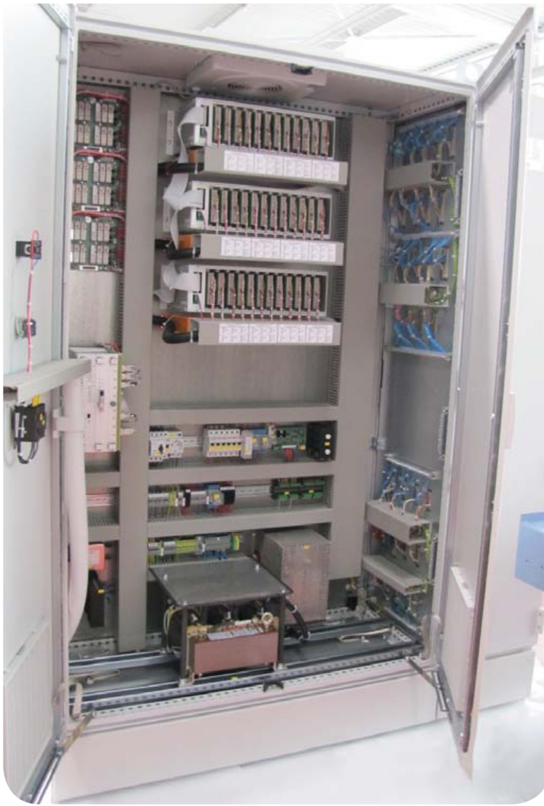
Neat and tidy: this (new) control cabinet still houses an original EPRO control (left). Each retrofit should also include new cables, depending on the system's age and condition. They could become brittle over the years and lead to faults in view of the harsh production conditions prevailing in glassworks
